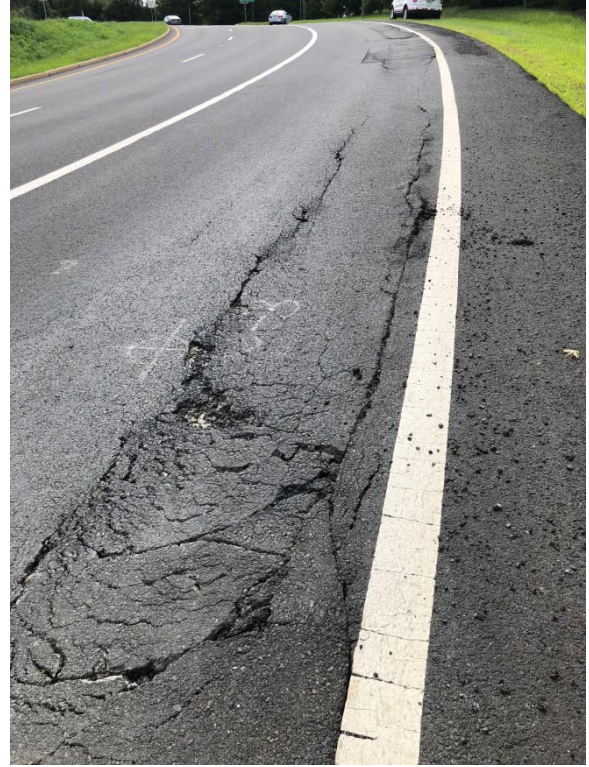
Photo 2: Example Deteriorated Pavement
